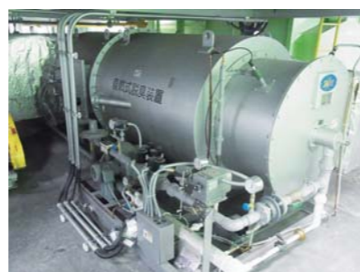
LPG burner for the drying furnace
