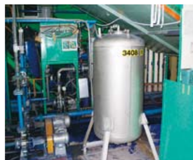
Cation resin tower
