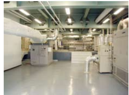
Dilution tunnel facility
