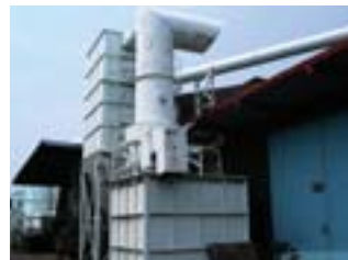
Casting process dust collector for electric melting furnace
