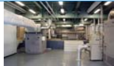
Dilution tunnel equipment
