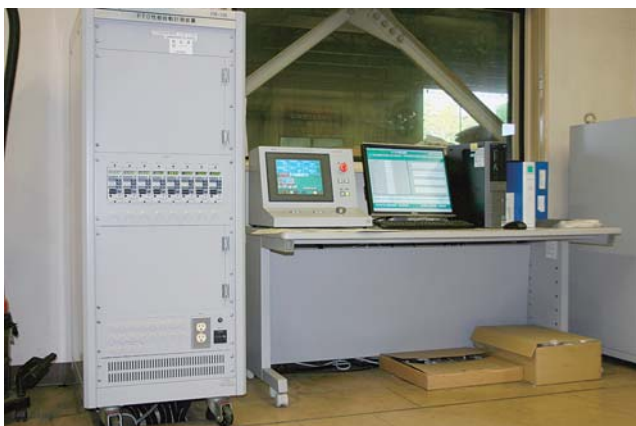
Operation measurement control panel
