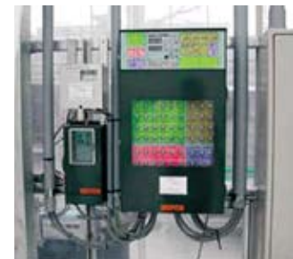
Integrated climate control system
